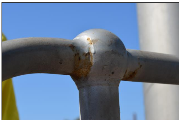
An example of poorly repaired handrail in a severe corrosive environment (wastewater treatment plant) where the repaired area has failed well before the main hot dip galvanized rails and posts.
