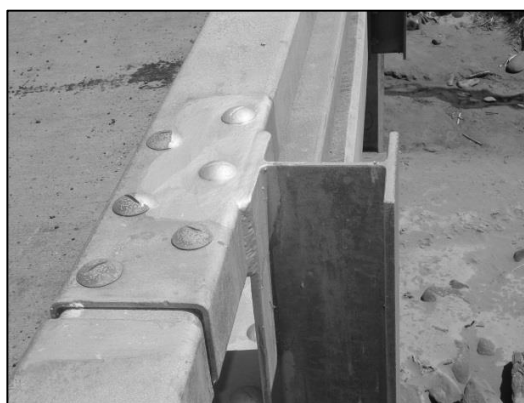
An example of well repaired handrail in a severe corrosive environment (marine).
