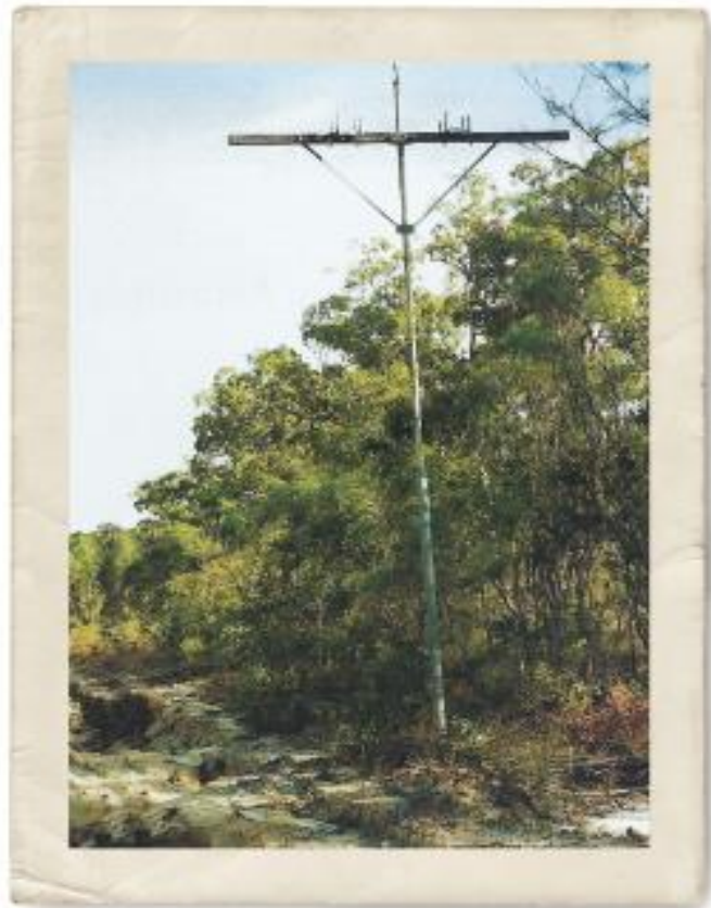
The original 1883 overland telegraph pole system was thought to have another 200 years of life left in the galvanizing when it was decommissioned in 1997.
